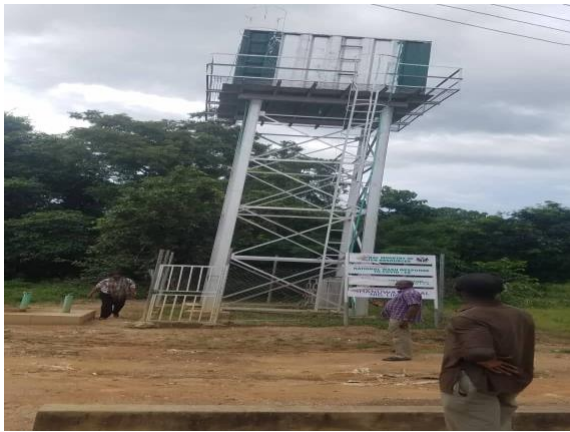
Kogi State Ministry of Water Resources in collaboration with the Federal Ministry of Water Resources Construct Solar Powered Industrial Borehole at Ikoja Odo Ere Community
