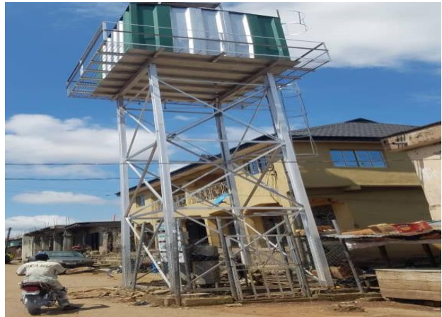
Kogi State Ministry of Water Resources in collaboration with the Federal Ministry of Water Resources Construct Solar-Powered Industrial Borehole at Madabo Community Lokoja
